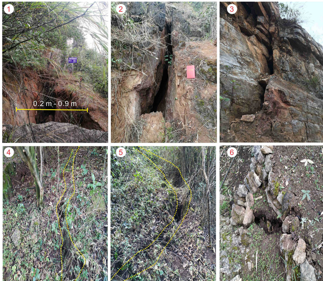
Fig. 5 Enlarged view of discontinuities and cracks found along the landslide scarp (orange line in Fig. 4e) before the 17 February 2019 rockslide. Yellow dotted lines show the cracks surrounded by vegetation
