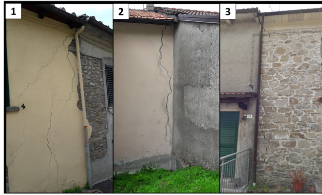
Fig. 7 Damage identified during the field survey of Carpineta hamlet. (1) Cracks in the external wall of a building in the central part of the village (sector 1). Front (2) and back (3) part of the same building affected by a vertical fracture in the southern part of the village (Sector 2)
