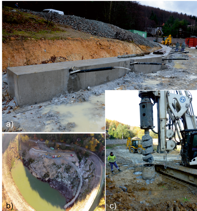
Fig. 14 a View of the anchored reinforced concrete wall. b Aerial view of remedial works in progress. c Drilling the piles
