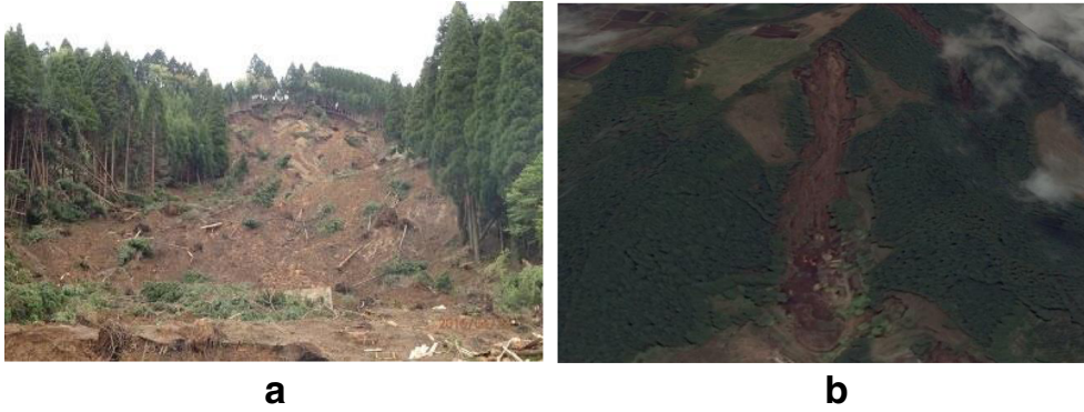
Fig. 6 Landslide at Hot Spring Resort (32.877°N, 131.016°E). a Field photo taken on April 23, 2016 by Kiyota Laboratory (Geo-Disaster Mitigation Engineering, http://www.gdm.iis.u-tokyo.ac.jp/index_e.html ), view to NWW. b Very high-resolution satellite image from DigitalGlobe on GE platform shot on April 19, 2016 in three-dimensional view, view to NWW
