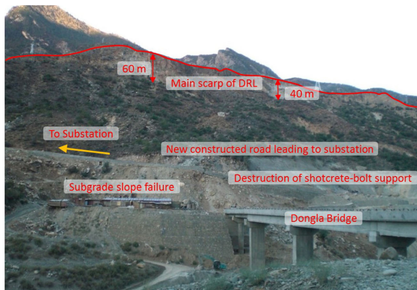
Fig. 6 Main scarp and local deformation features of the DRL. Viewing toward southwest
