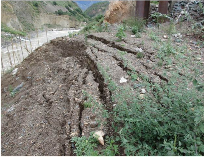
Fig. 17 New emerging arc tensile cracks on the artificial slope (photo taken February 2014)
