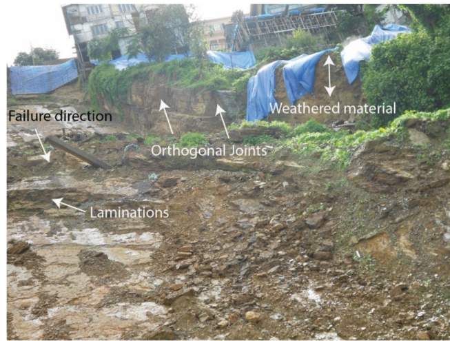
Fig. 9 Outcrop of the failed slope showing orthogonal joints, failure direction, and a layer of weathered and nonfissured clay on top
