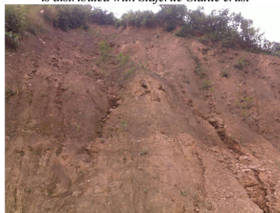
c Landslide occurred from completely weathered materials of a cut-slope in Quan Ba district, where is distributed with Ferrosialite crust
