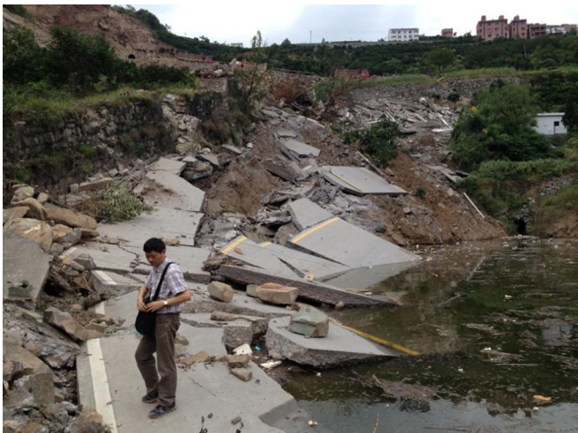
Fig. 7 View of the lower part of the Shanshucao landslide, road G348 was moved at great differential displacements, and the concrete pavement broken into pieces
