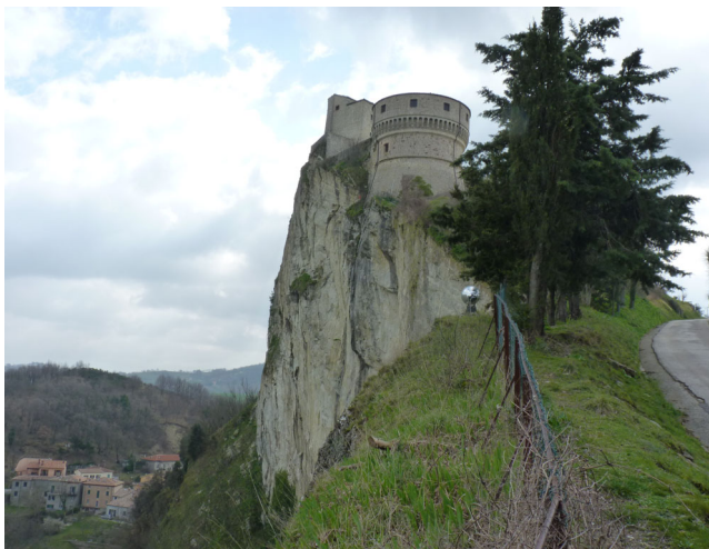
Fig. 10 Detail of the east-facing rock cliff beneath the fortress’ north tower. The vertical fracture developing below the tower is already open, as clearly shown by the presence of vegetation and debris in the upper part
