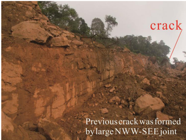
Fig. 9 Previous crack at back border of rockslide at Sanxicun (also see Fig. 8)
