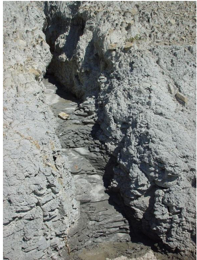
Fig. 11 Gully of more than 20 cm depth in the regolith developed on the surface of a 6-years old excavated slope of the C-25 road at Gurb, Spain (stage 4)
