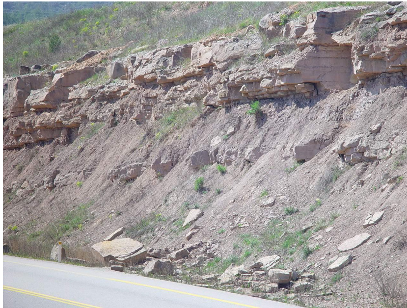
Fig. 3 Differential weathering along the C-16 road at Navàs, Barcelona province, N Spain. Spalling and disaggregation of the mudstone have generated overhangs in the sandstone layers which eventually fall
