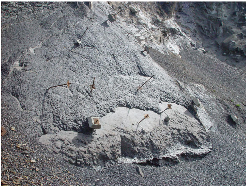
Fig. 2 Cut slope surface deterioration in the N-1 road at Ormaiztegi in the Gipuzkoa province, N Spain. The argillaceous rock decomposes around the bolt thus preventing its proper operation
