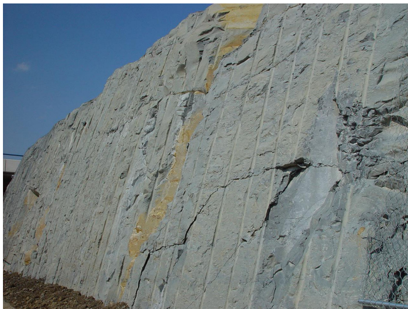
Fig. 4 Slightly deteriorated cut slope. Well-preserved blast holes are observable several years after the excavation of the slope in the C-17 road at Torello, Barcelona province, NE Spain
