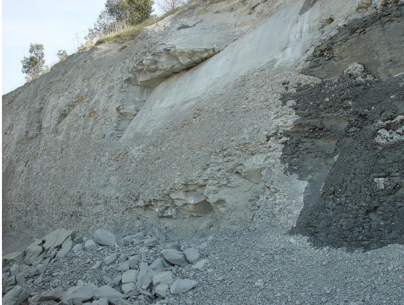
Fig. 1 Slope surface deterioration with the development of listric (curvilinear) failures on mudstones in the C-17 road at Tona, Barcelona province, NE Spain
