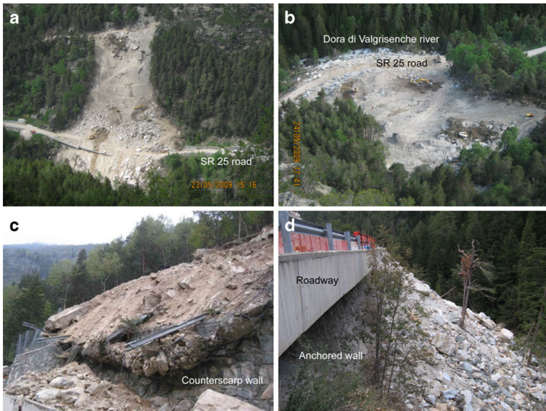
Fig. 2 a General view of the landslide (May 2009) from the opposite valley side. b View of the landslide (May 2009) from the crown area. c Detail of the counterscarp wall partially overstepped by the landslide mass. d Details of the SR25 roadway and anchored wall
