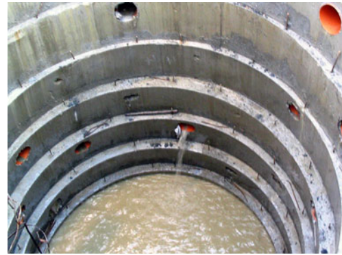
Fig. 14 Primary lining of the shaft at the Slano blato landslide during construction. The photo shows the drainage ability of the shafts/wells
