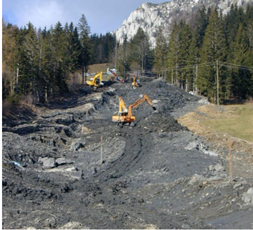
Fig. 12 Construction of the drainage trench in the middle section of the Macesnik landslide
