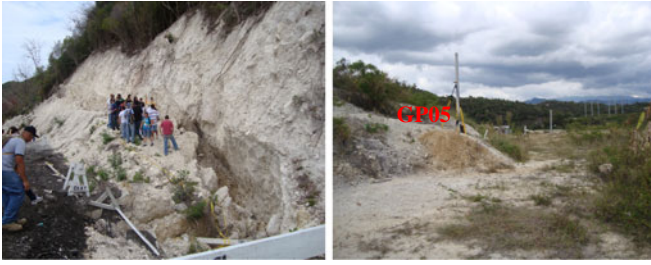
Fig. 3 Photos showing the head scarp (left) and the toe area (right) of the landslide
