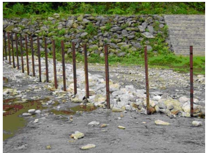
Fig. 26 Vertical steel bars to retain trees and vegetation
