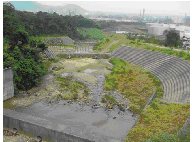
Fig. 25 Gabions with reinforced shotcrete protecting the lateral dyke between the B-5 and the BS-1 dams
