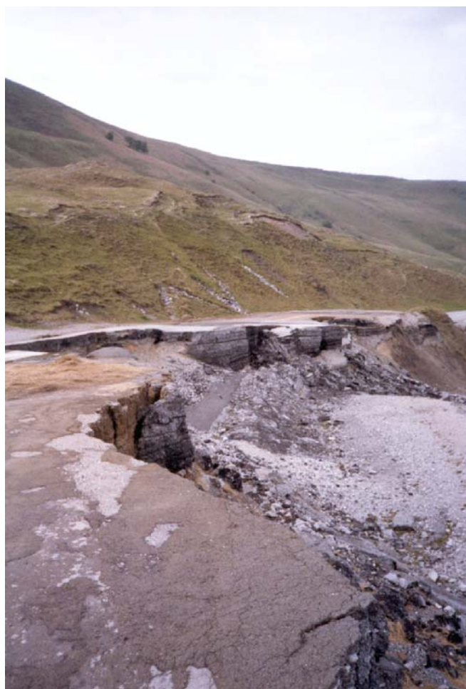
Fig. 4 Photograph of a section of the upper road showing multiple phases of road repair, and movements that have occurred since the road was closed in 1979
