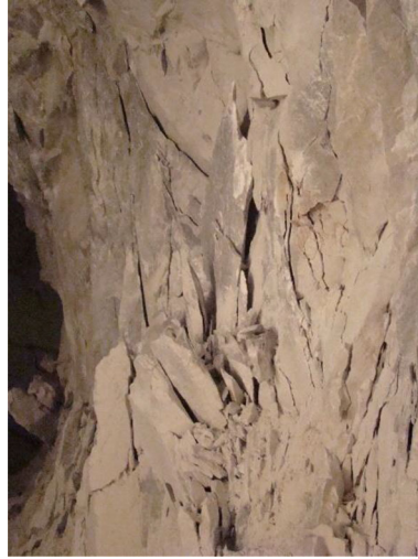
Fig. 5. Fracture and bulging of side wall F in first-phase test tunnel in Jinping Underground Laboratory
