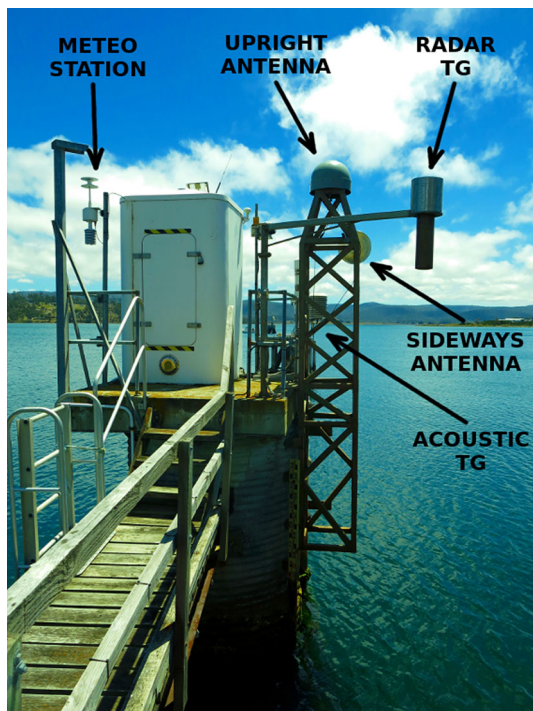
Fig. 2 Northward view of the Spring Bay site, Australia. The labels indicate the location of each instrument. The air gap distance from the acoustic TG to the mean sea-level surface during the experiment is approximately 3.6 m
