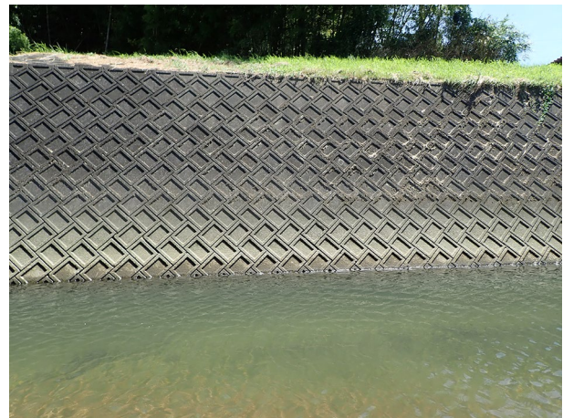
Fig. 2 Concrete revetment along shoreline in the tidal reaches of Kedo River on August 13, 2018
