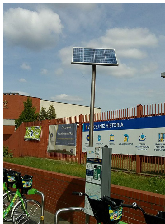
Fig. 9 PV micro-system powering the bicycle control panel, Toruń (photo: B. Igliński)
