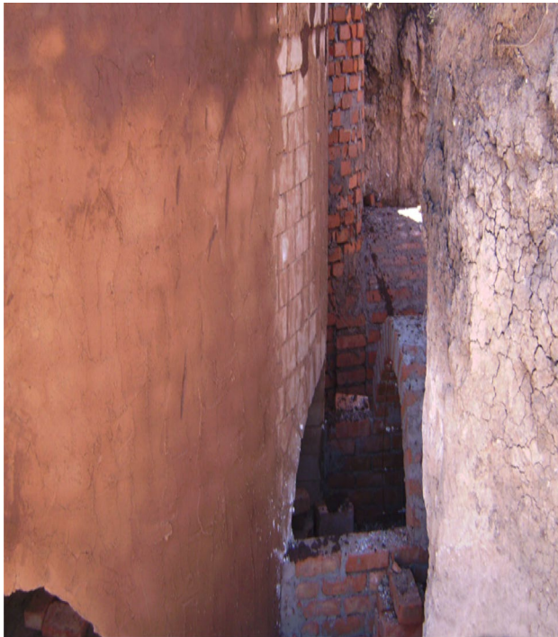
Fig. 2 Coupled kilns duct to drive the combustion gases with adobe as external insulation
