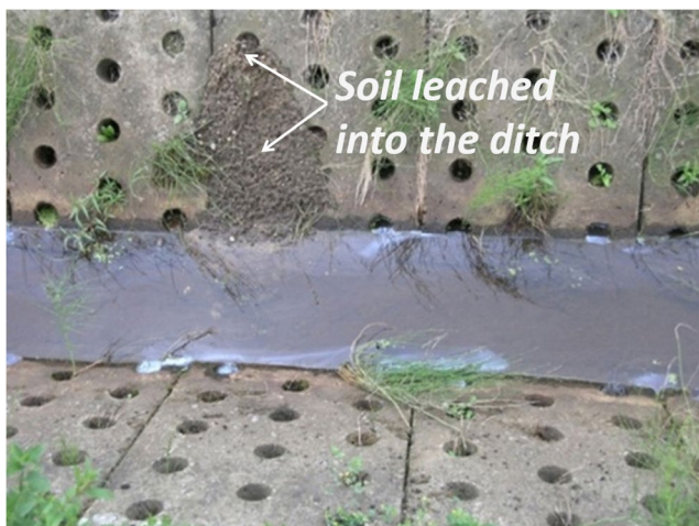
Fig. 6 Soil erosion observed in the ditch of the dam
