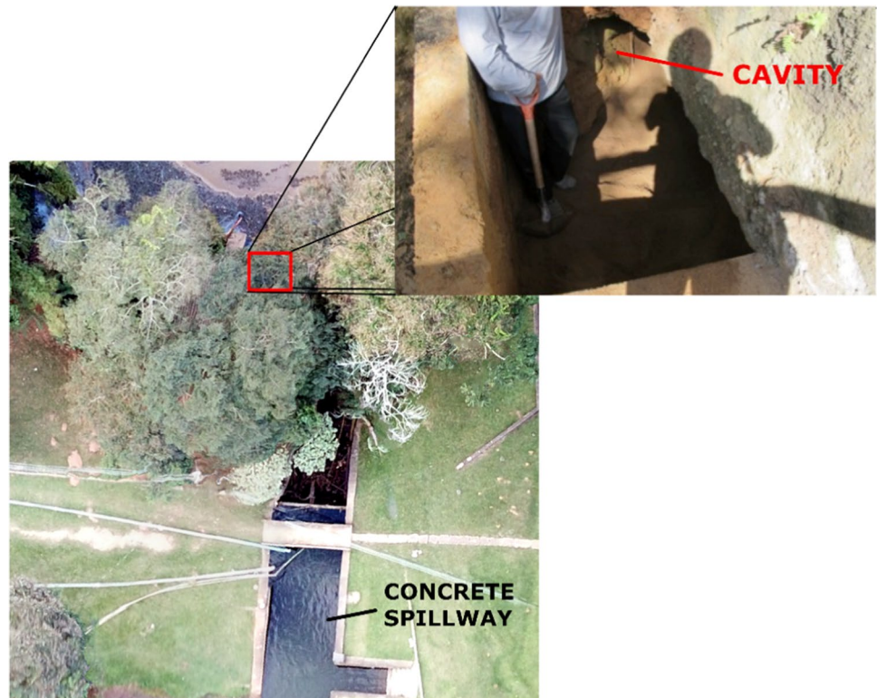
Fig. 3 Location and detail of the erosive cavity caused by piping on the downstream slope (adapted from Minette 2015)
