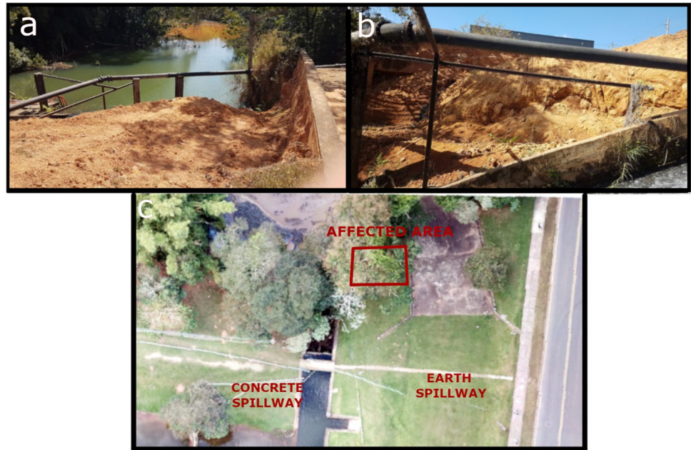
Fig. 13 Register of the landslide occurred on the downstream slope of the embankment. a) Upstream view; b) Downstream view; c) Top view of the dam highlighting the affected area
