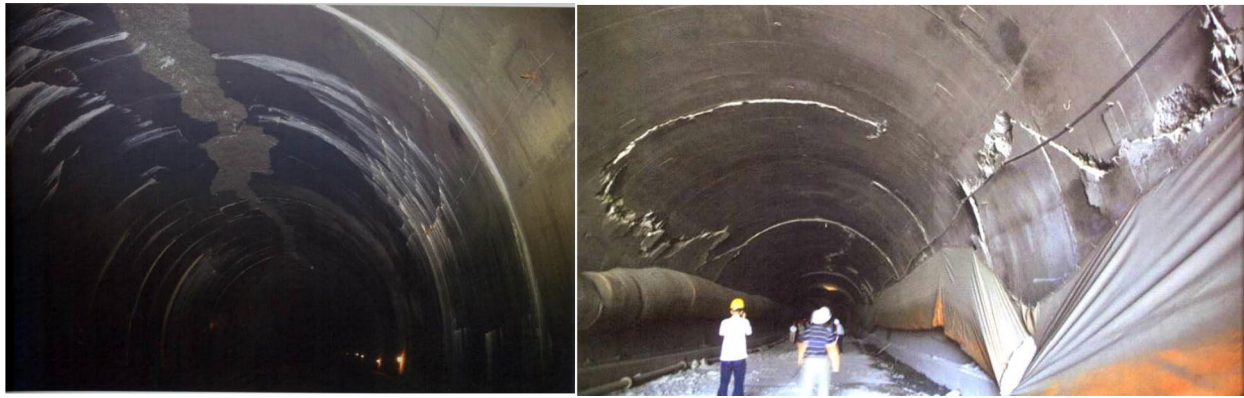
Fig. 1 Earthquake damage in cross-fault tunnels (Yu et al. 2016)
