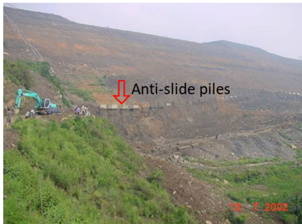
Fig. 2 Anti-slide piles exposed after a slide occurred in July 2002 (mirror to upslope)
