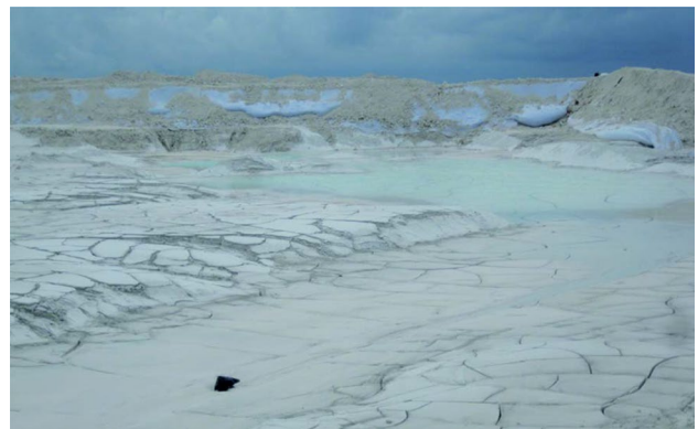
Fig. 2 Desiccation cracking phenomenon of coral clay foundation in calcareous sand filling site in Saudi RSGT project (Qin et al. 2021)
