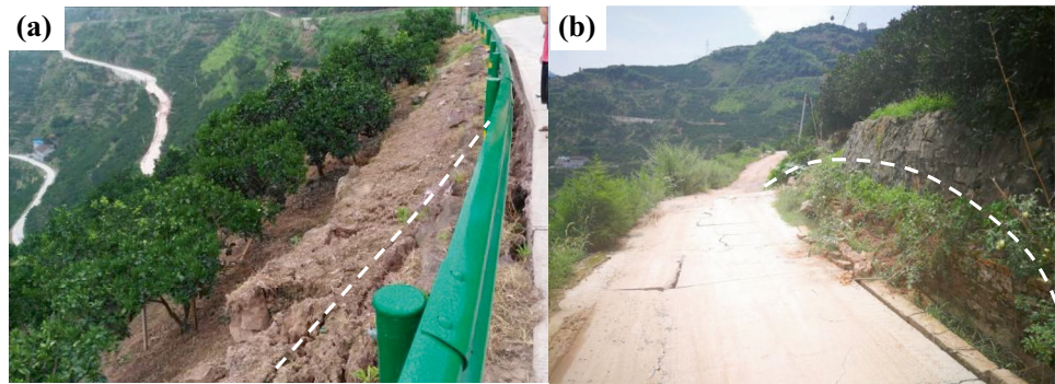
Fig. 8 Landslide deformation caused by rainfall in 2018: a crack LF3 outside the highway in the middle of the landslide, b crack LF4 in the highway retaining wall at the front of the landslide
