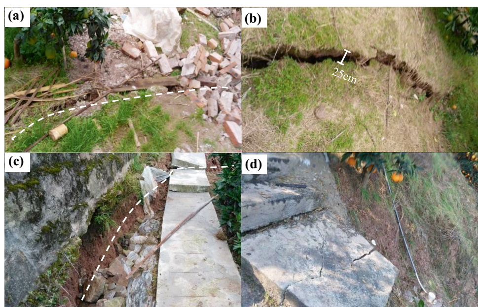
Fig. 7 Deformation of the middle part of the Tanjiawan landslide owing to autumn rain in West China in 2017: a damage to houses caused by the deformation, b crack LF2 approximately 80 m long, c road damage caused by the cracks, d damage to the cement board due to the deformation of the sliding mass
