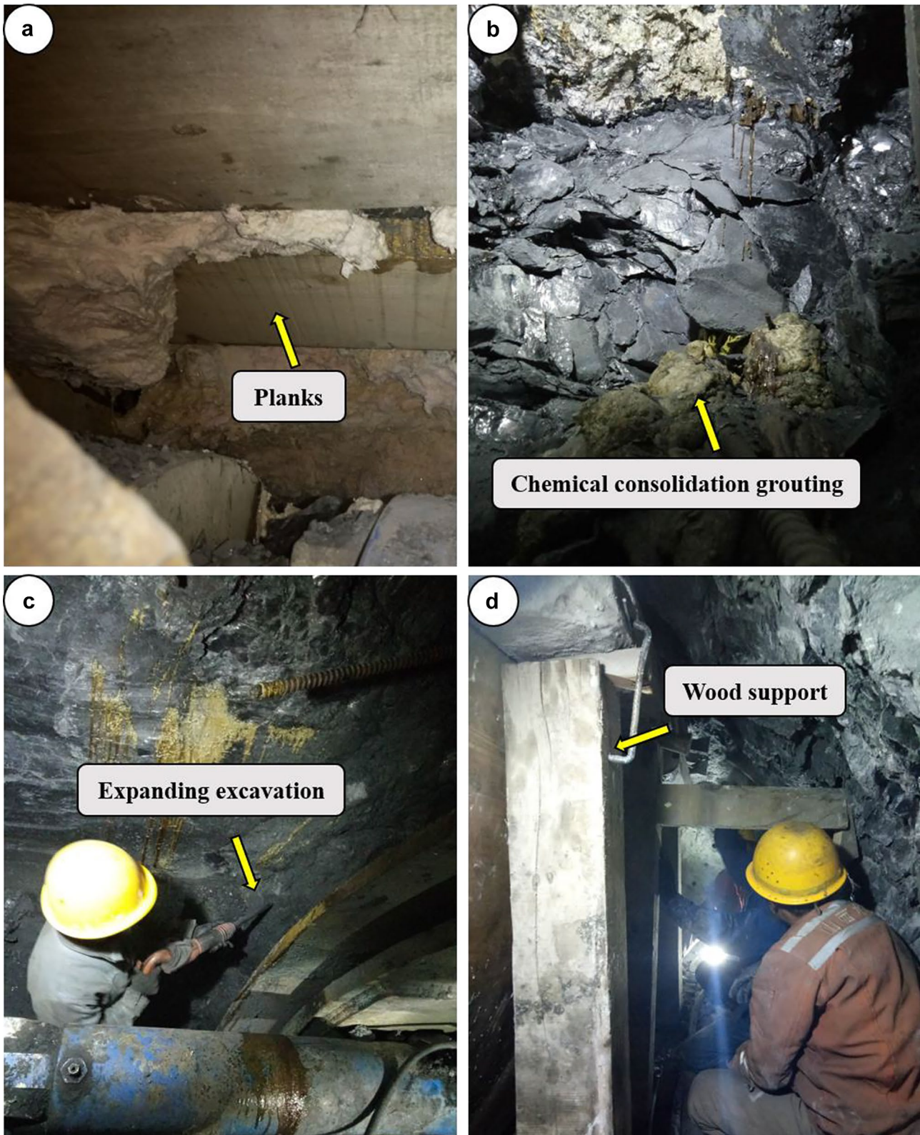
Fig. 15 Engineering treatment measures adopted for releasing TBM. a Supporting the collapsed cavity port with planks. b Chemical consolidation grouting. c Expanding excavation on both sides of the shield. d Supporting the pilot tunnels with square pieces of wood
