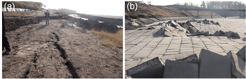
Fig. 2 a Representative failed canal slope and the b crushing failure of concrete slabs on the canal bed
