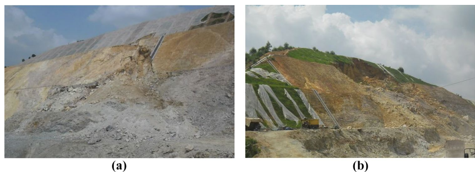
Fig. 5 Development of the slope sliding area from May to June 2015
