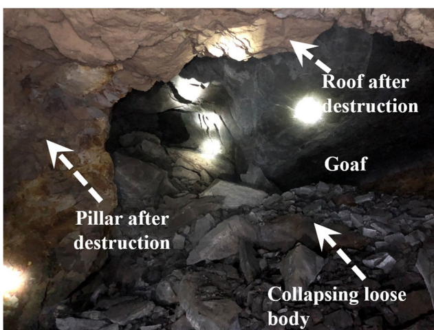
Fig. 14 Image of collapsed goaf
