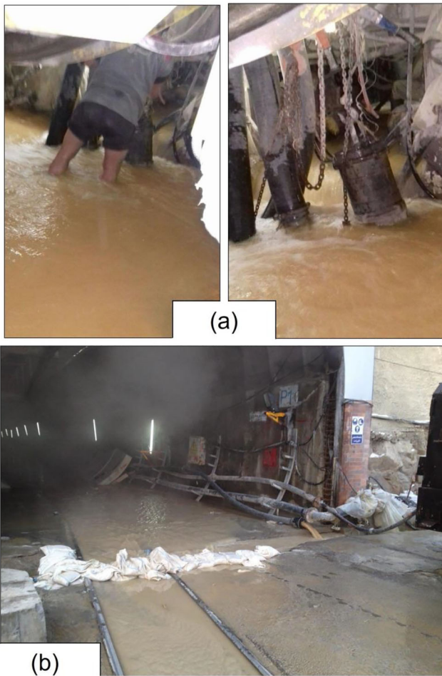
Fig. 23 Water inrush to a TBM Back up utilities, and b the tunnel outlet
