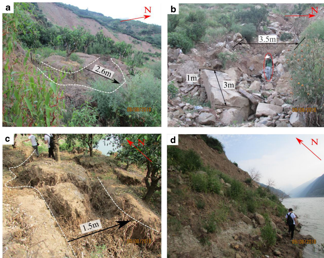
Fig. 8 Surface deformation behavior of the Yanguan landslide: a tensile cracks near the right flank of the landslide; b the gully near the left flank; c tensile cracks in the foot of the landslide; d the toe of the landslide
