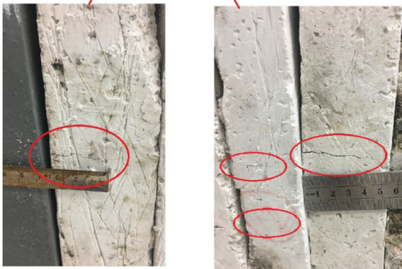
Fig. 4 Crack initiation stage and non-through cracks
