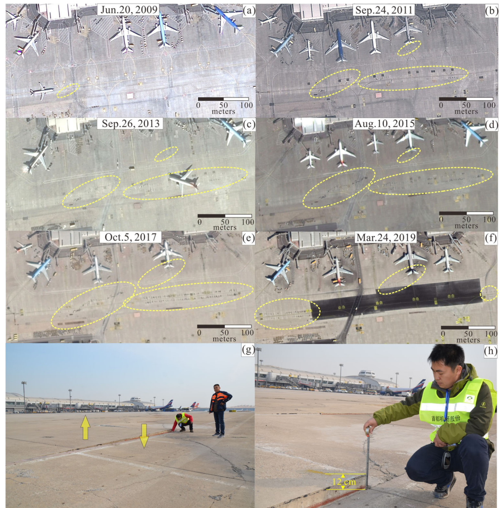
Fig. 12 Cracked cement concrete slabs and subsided southeastern side in the BCIA. Fissures are 300-m long, 1~10-cm wide, and have 1~12-cm vertical dislocations. Location is shown in Fig. 10. a~f Pictures are based on Google Earth image. g~h Photos were taken on March 15, 2017
