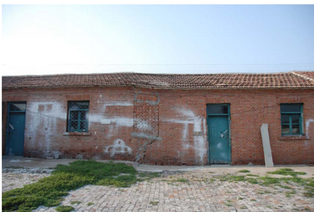
Fig. 5 Damaged building and floor in Tugou village (derived from the Beijing Hydrogeological and Engineering Geological Survey 2007). Location is shown in Fig. 4. The lens is aimed at north, and the right side has subsided
