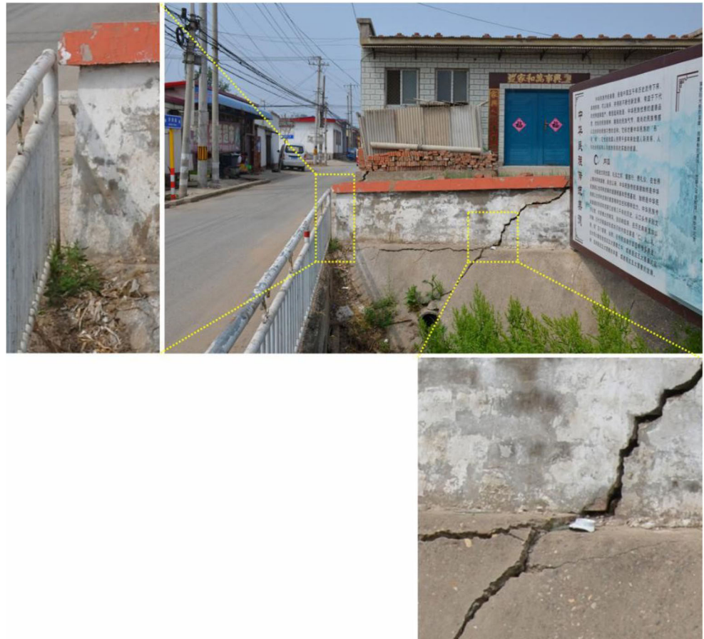
Fig. 19 Cracked house, wall, and dike with small vertical offsets in Beicai village. Photos were taken on May 16, 2018. Location is shown in Fig. 17. Fissures trending N10°E mostly covered by new concrete pavement. Wall tilted inward by fissure propagation
