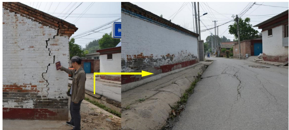
Fig. 18 Cracked house and pavement, without a measurable vertical offset, in Beicai village. Photos were taken on May 16, 2018. Location is shown in Fig. 17. Fissures in the pavement, trending E-W, 10~20-m long
