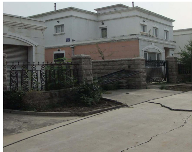
Fig. 6 Damaged roads and Villa 0702 in the Baxian villas (derived from the Beijing Hydrogeological and Engineering Geological Survey 2014). Location is shown in Fig. 4. Southeastern side has subsided
