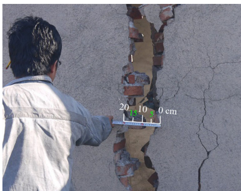
Fig. 5 Severe damage to a building wall
