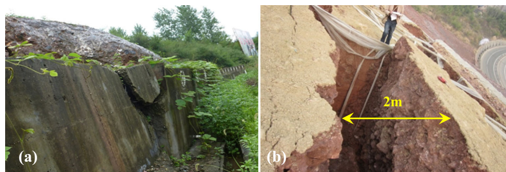
Fig. 3 a Local fracture on the concrete retaining wall; b characteristics of the deep tension crack
