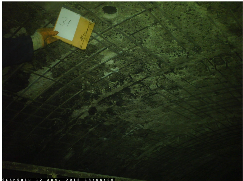
Fig. 8 Spalling of concrete and exposed reinforcement due to heat damage in the roof of the tunnel
