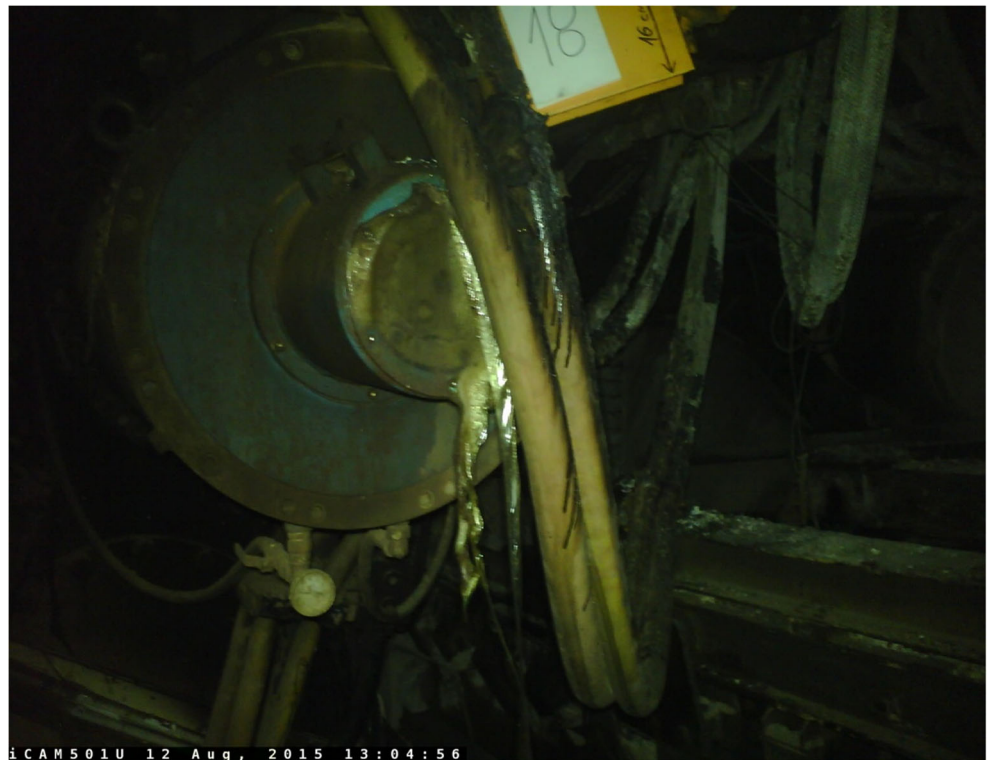
Fig. 7 The state of the cutterhead motor after the methane flare
