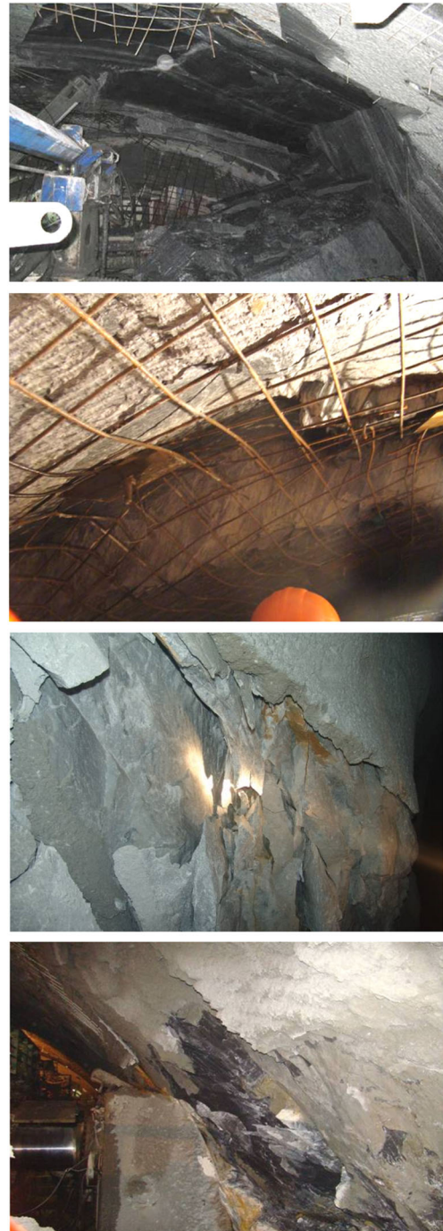
Fig. 6 Type of damage to the surrounding rock in a TBM tunnel
