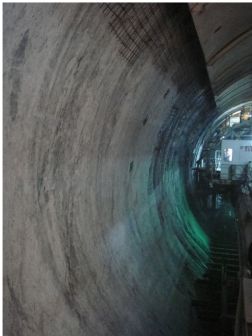
Fig. 4 An image showing that the wall is smooth in the tunnel excavated with the tunnel boring machine (TBM)
