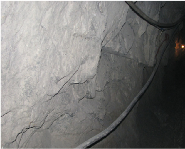
Fig. 3 An image of a clearly observable joint in the tunnel excavated using the drilling-blasting method
