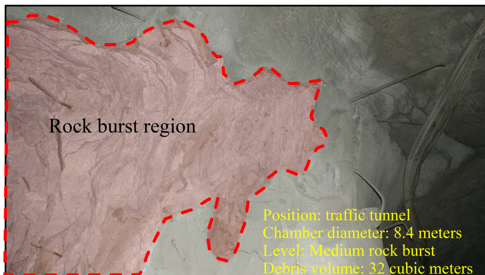
Fig. 4 Typical rock burst in the traffic tunnel
