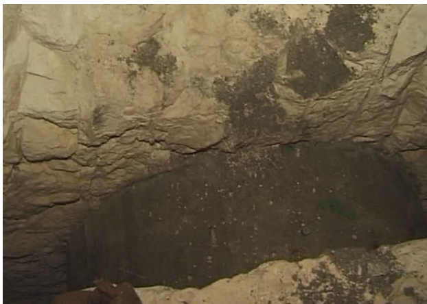
Fig. 3 The slot in the rock mass where a hydraulic jack was installed and concrete fill placed (example from the investigation works at the Komarnica Dam, Montenegro)
