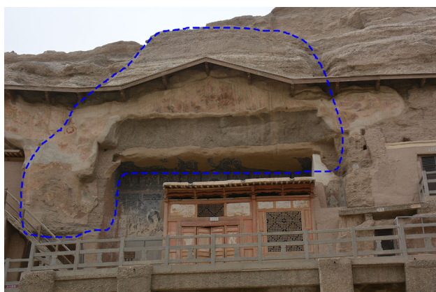
Fig. 4 Potentially dangerous body on the cliff. The dotted line indicates the area on the cliff with potential risks
