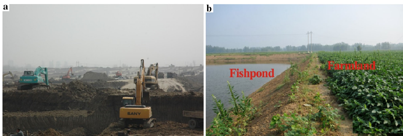
Fig. 7 Subsidence reclamation during (a) and after (b) excavating deep zones and raising peripheral areas
