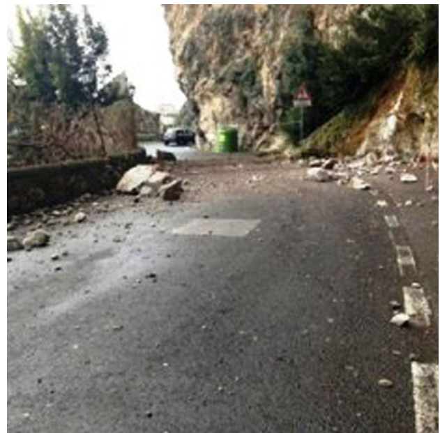
Fig. 11 Small size boulders fallen at the progressive kilometer 26 + 430, on 14th January 2014
