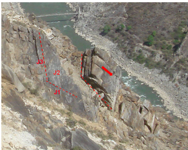
Fig. 4 Loose rock blocks observed in subarea B
