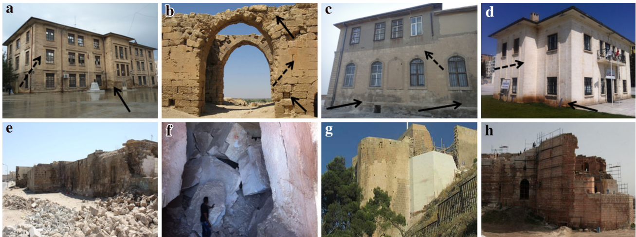
Fig. 4 Photographic evidence of (a–d) stone erosion that occurred on the roofs and in the bases of the masonry walls, (e–f) the structural damage, and (g–h) incompatible restorations
