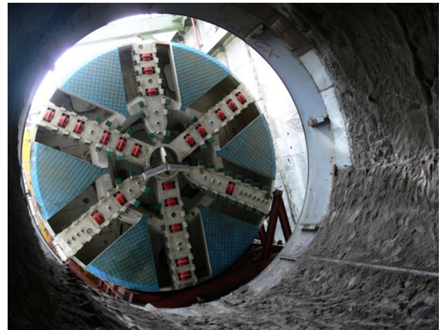
Fig. 2 Full-face view of TBMs used in the excavation of Tabriz metro line 1
