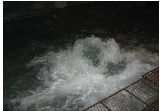
Fig. 14 Groundwater inflow at CH.11240 m in headrace tunnel 3
