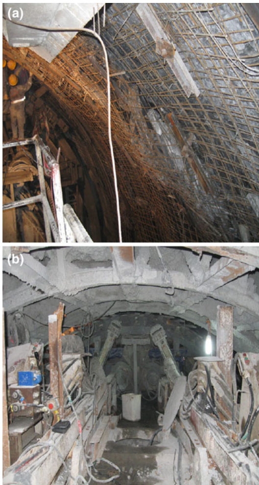
Fig. 10 a Support at unstable section b steel arch and structural support at rockburst section
