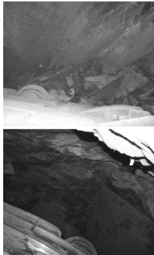
Fig. 6 Examples of tunnel face collapse
