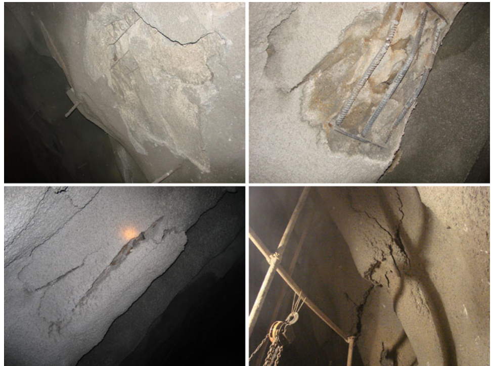
Fig. 6 Failure of the lining shotcrete at the right foot of the arch crown
