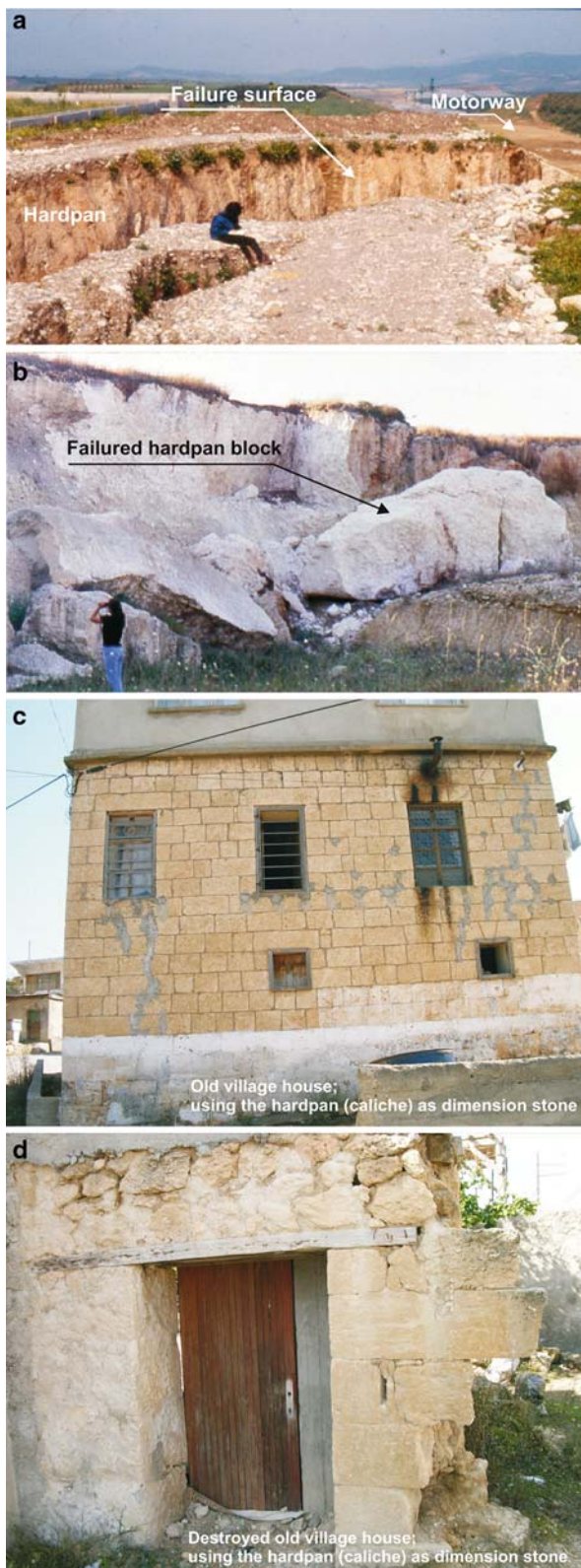
Fig. 2 a Motorway slope failure in caliche deposits, b mass movement in caliche deposits, triggered by 1998 Adana–Ceyhan earthquake, (c, d) the use of caliche hardpan as a dimension stone
